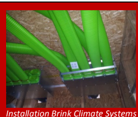
Installation Brink Climate Systems
